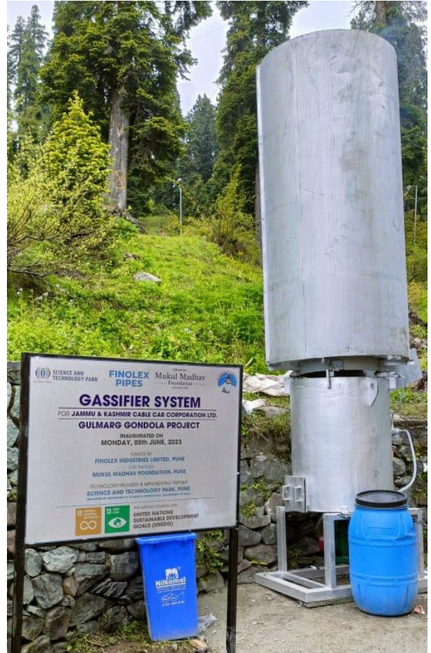
Gasifier system installed at the popular Gondola Ride site, Gulmarg, Jammu and Kashmir .
